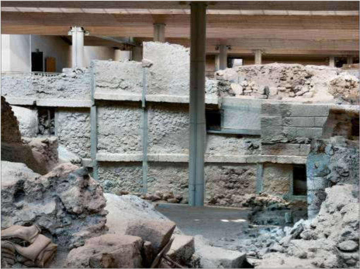
North view of Xeste 2 with the prominent string courses of dressed blocks of tuff.
