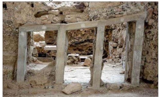
Polythyron in the ground floor of the east wing of Xeste 3. Its frame, distorted due to the decay of the timbers, was replaced with reinforced concrete in the course of its excavation by Spyridon Marinatos.
