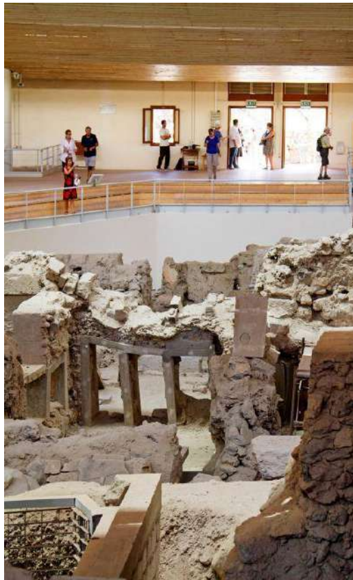
Polythyron in the ground floor of the east wing of Xeste 3. Its frame, distorted due to the decay of the timbers, was replaced with reinforced concrete during its excavation.
